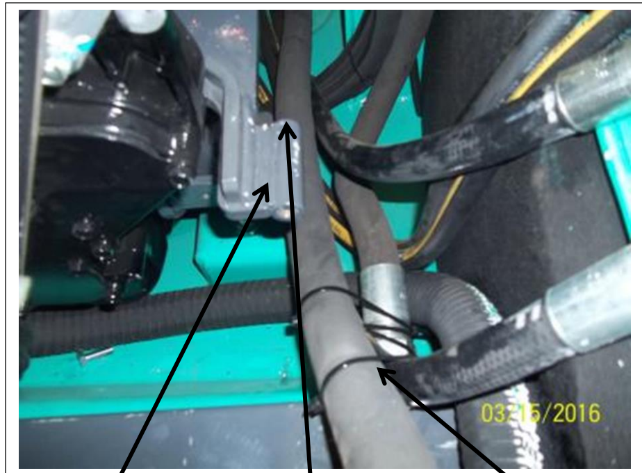
Compressor will mount here.
